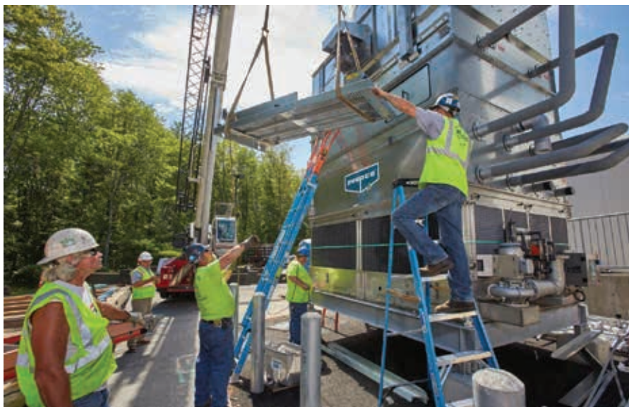
From top: The New England BioLabs facility under construction. > New EVAPCO cooling tower modules are prepared for installation.
